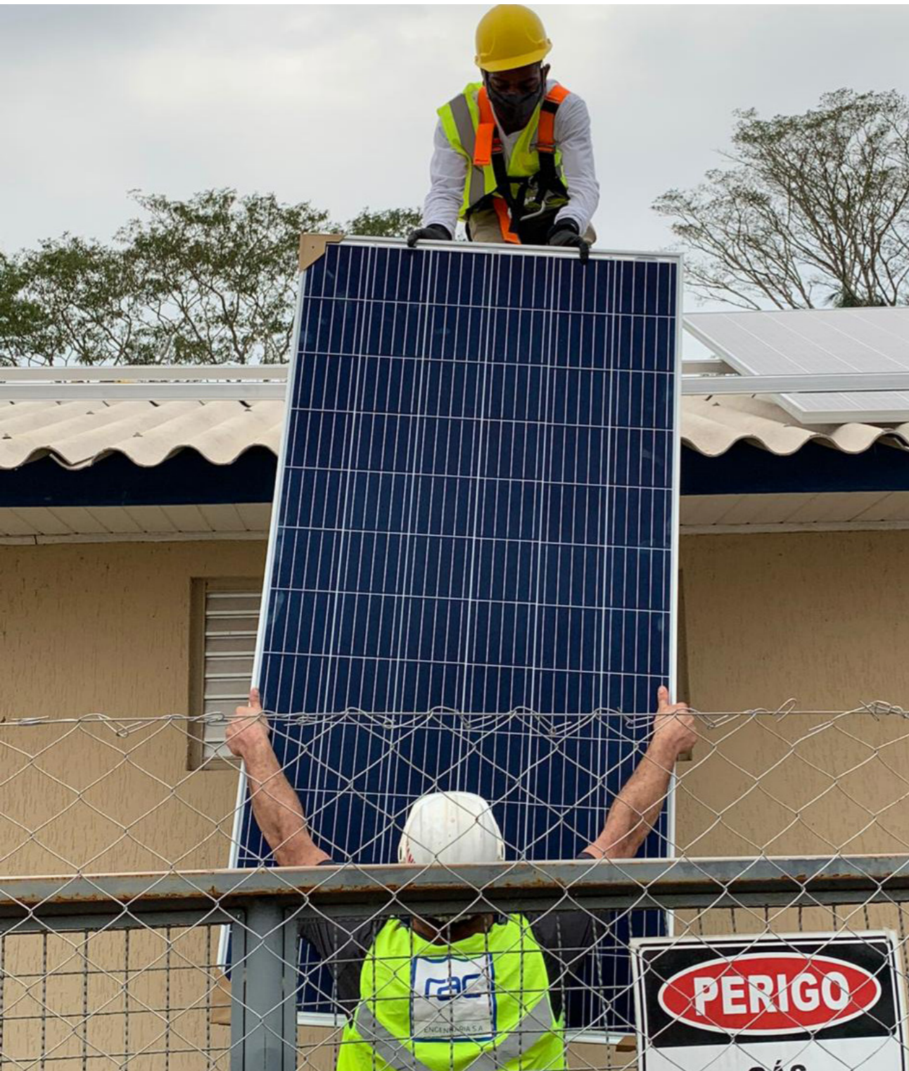
Photovoltaic Plate ETE Ouro Verde - Photographer: Alexandre Moreno Lisboa
