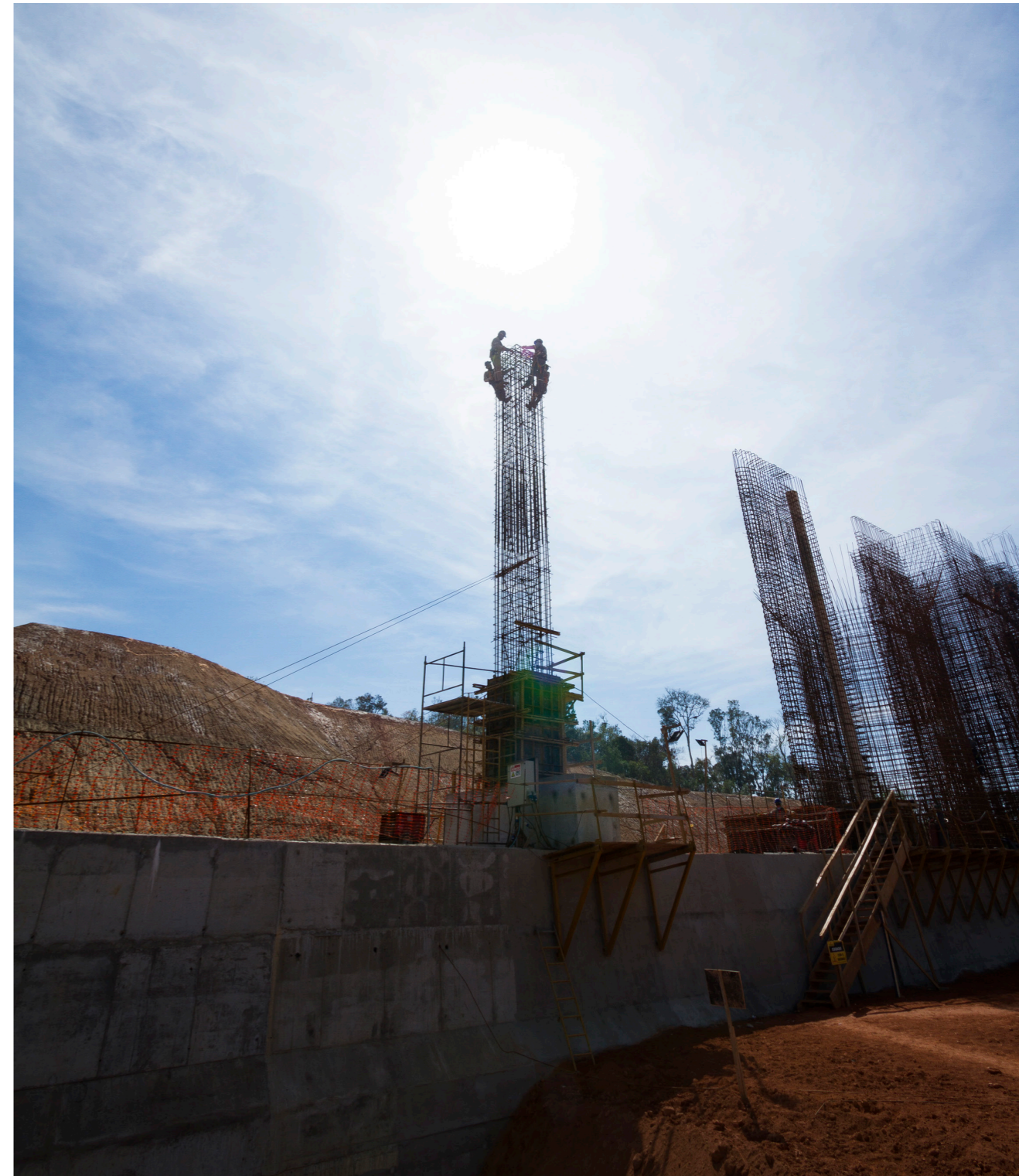
Miringuava Dam Work - Grading of the Tulipa structure –Photographer André Thiago Chaves Aguiar
